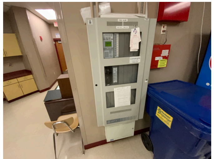
28 - FIRE ALARM PANEL
